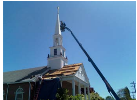
Rob Soave's roofing crew at work, along with T-Mobile's antennae installation prep team
